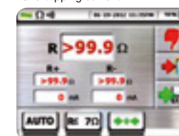
Continuity of protective conductors: Measurement result negative
